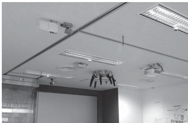
Photo 2 State-of-the-art facilities are installed above ceilings and behind walls.
