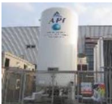
Nitrogen supply system
