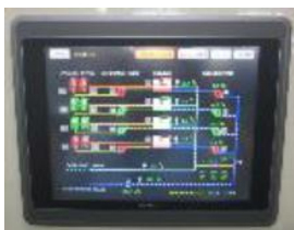
Air conditioning equipment control panel
