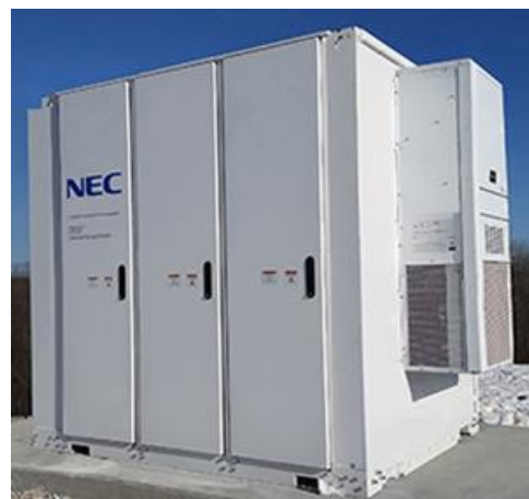
Medium-size self-contained energy storage battery system
