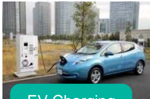
EV Charging Infrastructure
