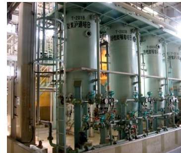
Circular effluent facility
