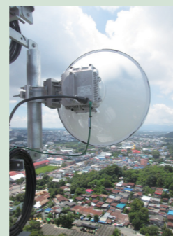
An iPASOLINK established in Thailand's Nakhon Sawan Province
