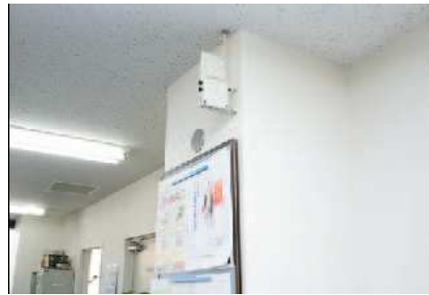
Example of installation of Access Point
