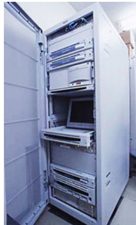
▲ With its outstanding flexibility to address future business development, NEC Express5800/420La (accommodated in the enclosures at the bottom inside the rack cabinet) supports the consolidated product master control system. Two of the storage appliance server iStorage/NS400 are located at the top inside the cabinet.
