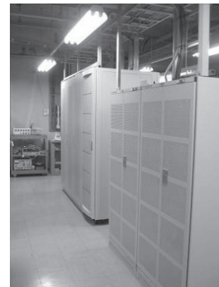
Photo 3 Terminal equipment (JMA).
